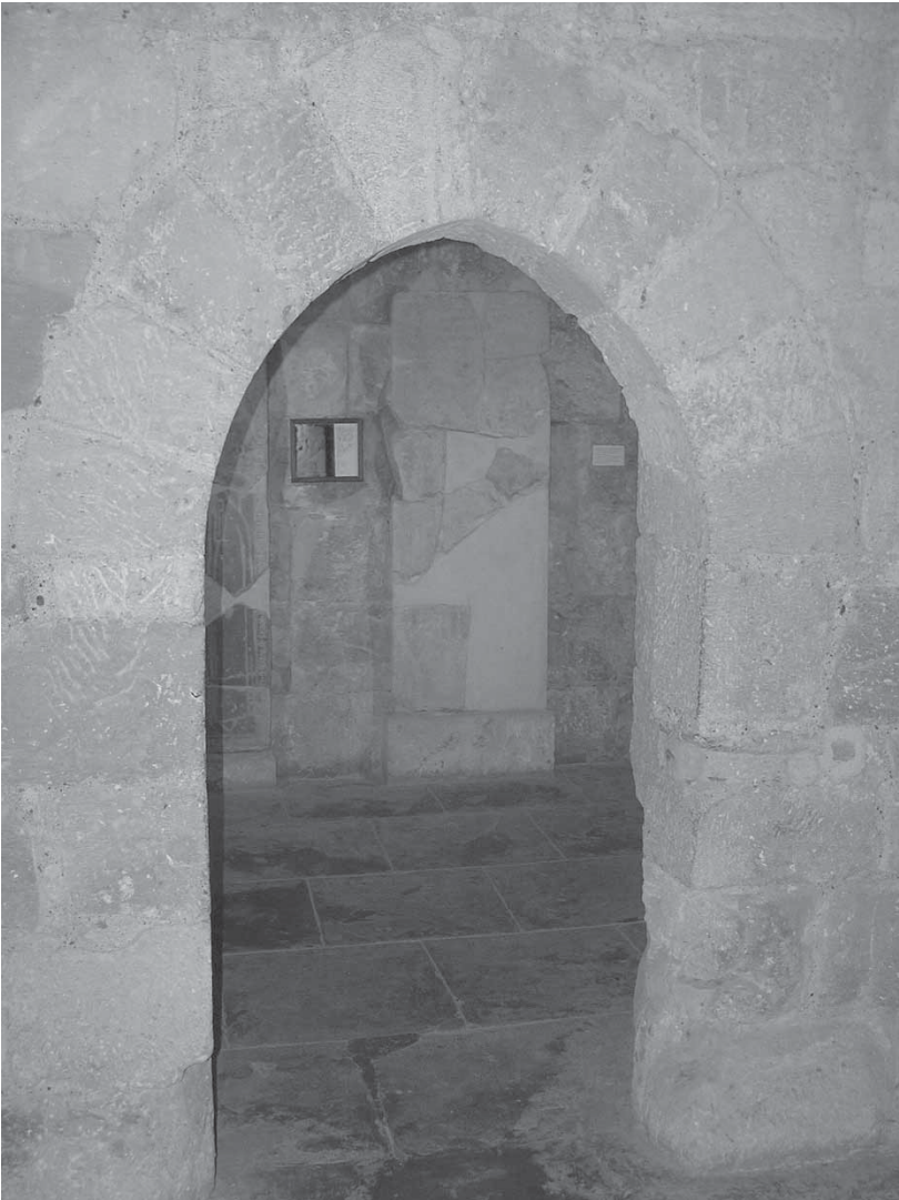
Fig. 28: Limassol Castle, lower level of cells, restored masonry in cell portal [M. Olympios].
